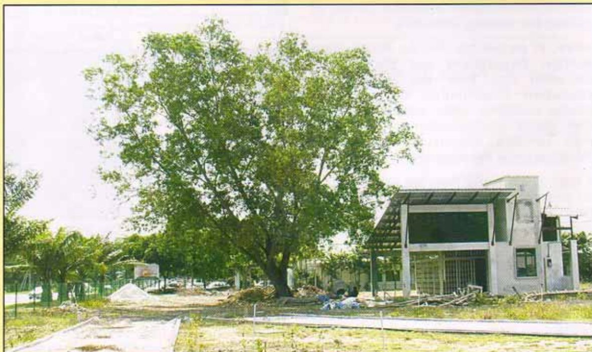
▲ The almost completed Daybreak Landscape Gallery shop building and its surrounding walkways.
